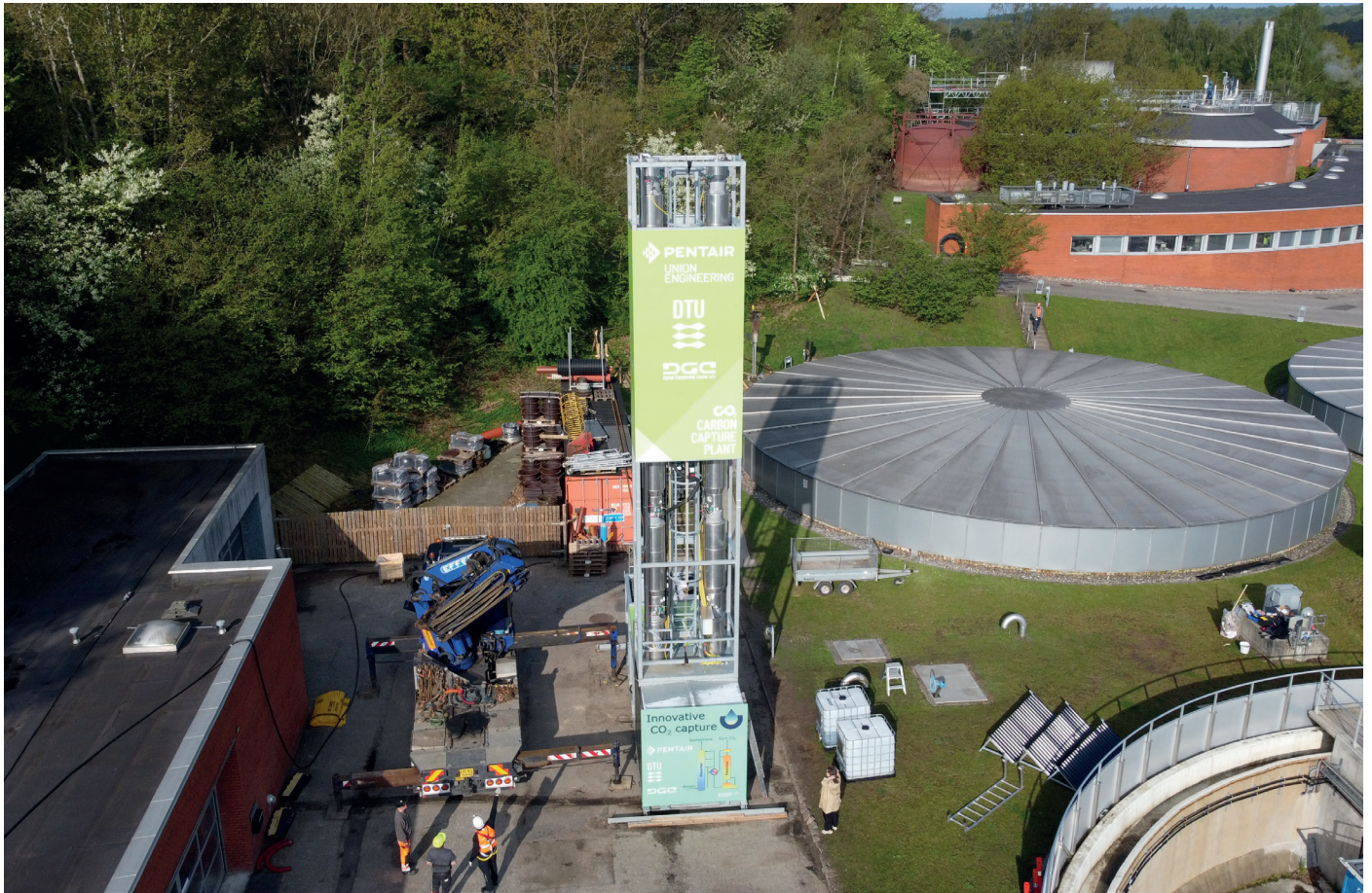
Mobile carbon capture unit at the public sewage treatment plant Mølleåværket
