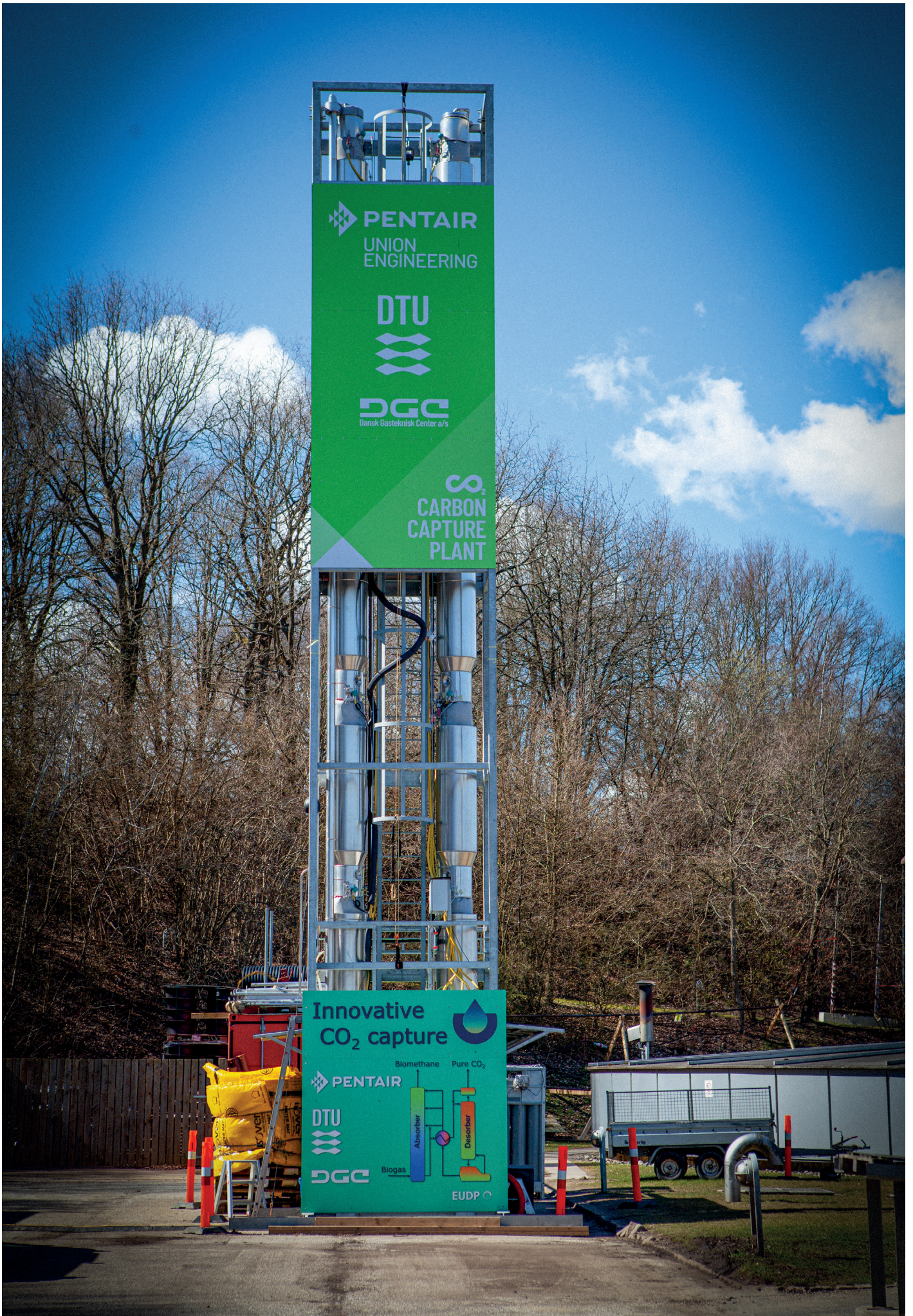
Mobile carbon capture unit at the public sewage treatment plant Mølleåværket
