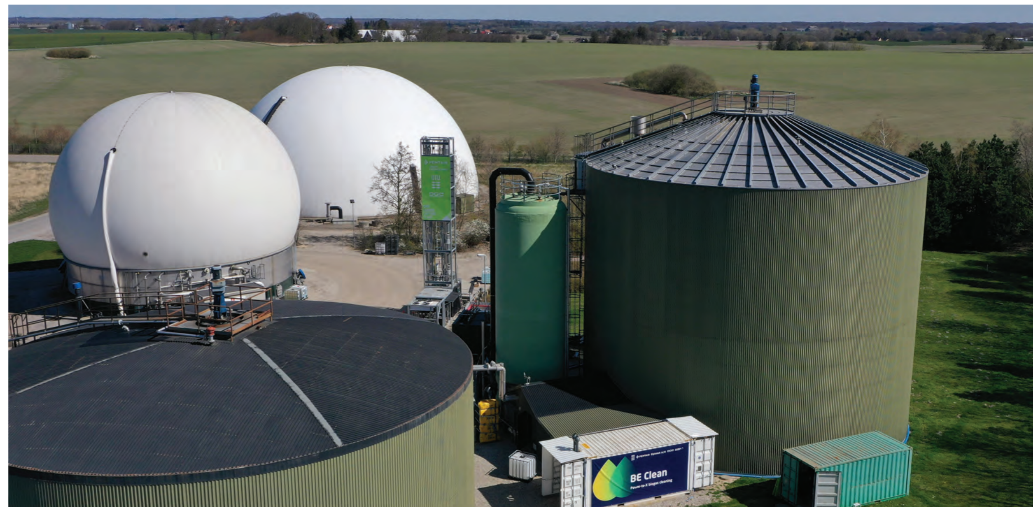
Carbon capture and PtX biogas cleaning demonstration plants at Hashøj biogas. The green tower in the back is the DTU carbon capture pilot plant that is part of the BioCO 2 project, and the container with the blue banner in front is part of a Power-to-X gas cleaning project called BE Clean
